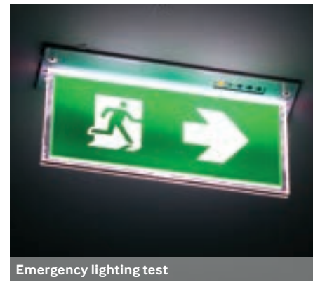
Emergency lighting test
