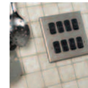
Appliance control panel
