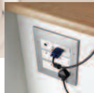
Multimedia control panel
