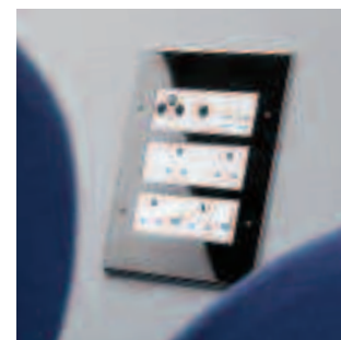
Multimedia control panel
