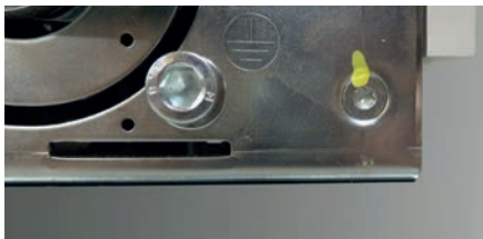
Connection point on the fixed DMX 3
